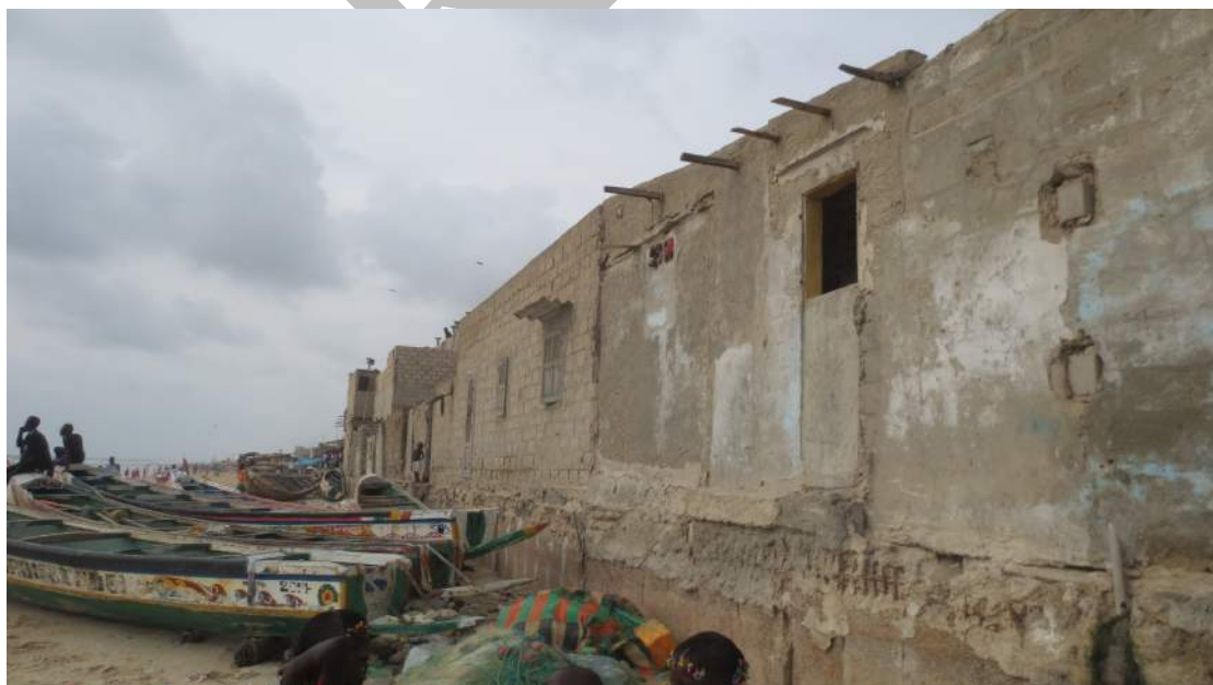
Figure 1: Partially destroyed home in Guet Ndar, Saint-Louis 5
